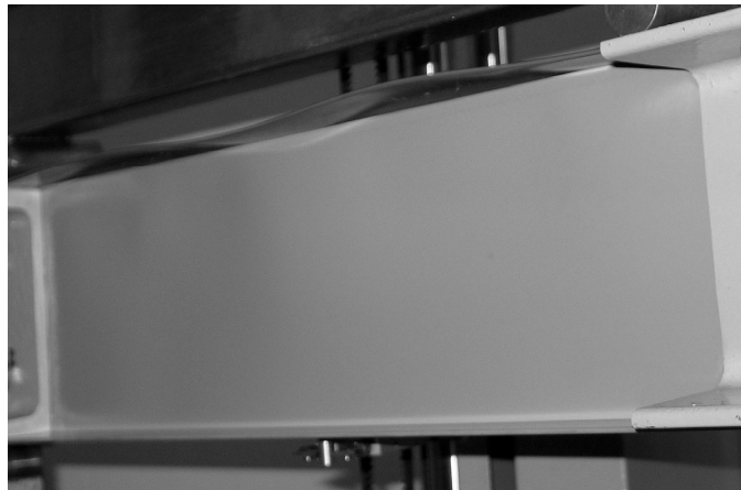
Fig. 4. General view of the beam with buckled flange (Fot. M. Ostwald)
