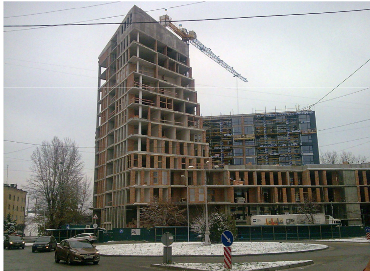
Fig. 5. The construction site view on November 22, 2018, after all storeys erection in the three sections of the residential complex.
