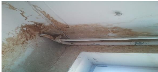
Figure 4 – The microbiological corrosion in industrial building
