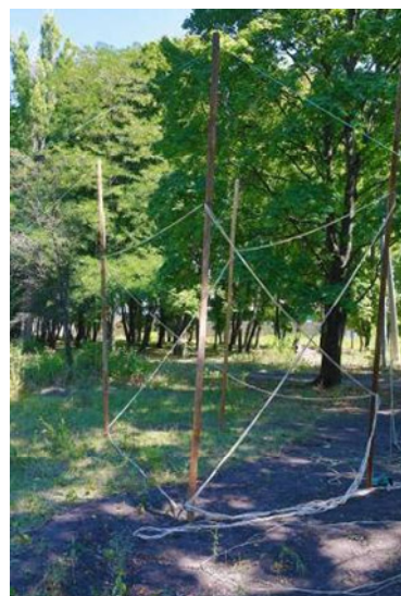
Fig. 3. Location of three compensating windings of experimental plant of system of active shielding
