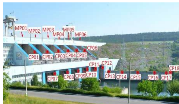
Fig. 12. Reflector sites CP01-CP18 determined by linear-angular methods and GNSS sites MP01-MP06 (view from point DSR1)
