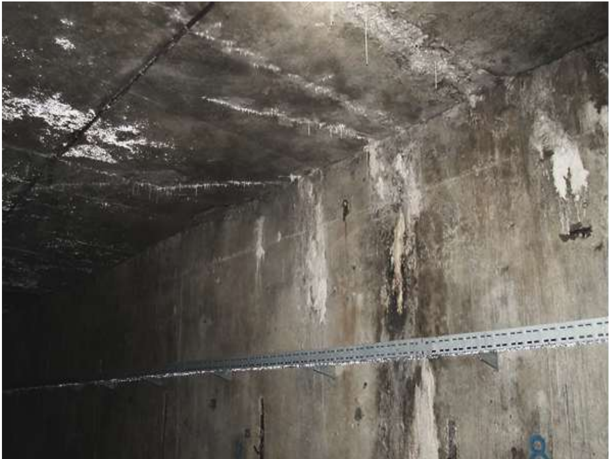
Figure 1 - Cracks with filtration in a concrete timbering of gallery of the Dniester hydroelectric power station
