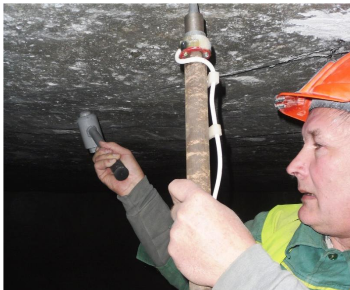
Figure 4 – Realization of vibroacoustic diagnostics of a roof of development by basic option
