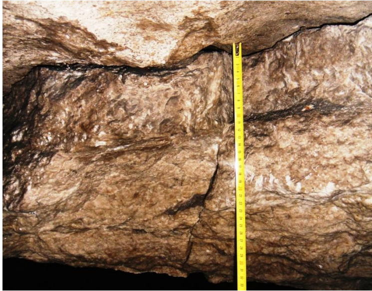
Figure 3 – A photo of separation in a roof of the main transport gallery
