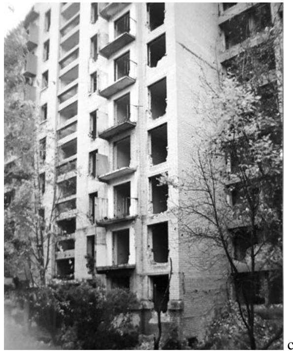
Figure 7 c - Deformations of buildings along the eastern side of the Monastirskyi gully
