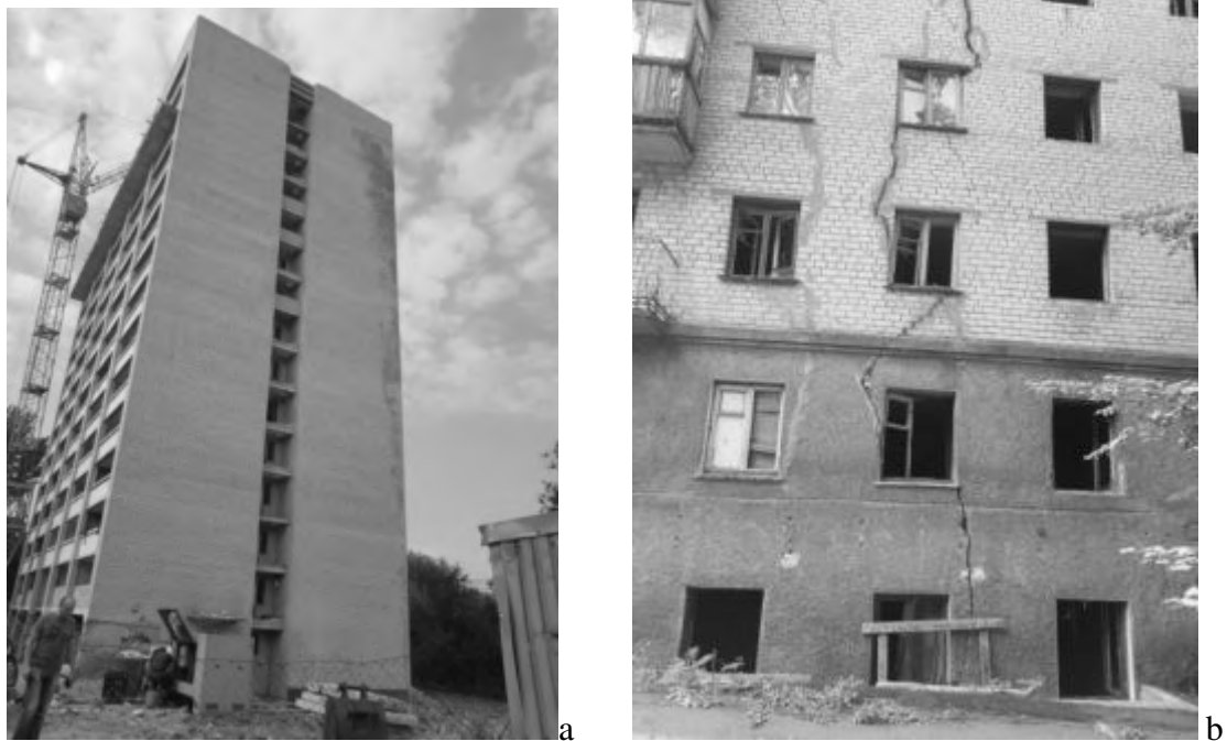
Figure 7 - Deformations of buildings along the eastern side of the Monastirskyi gully
