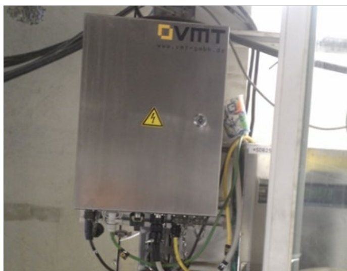
Figure 9 – Central Radio Modem (Switch). (Tashkent-2018)
