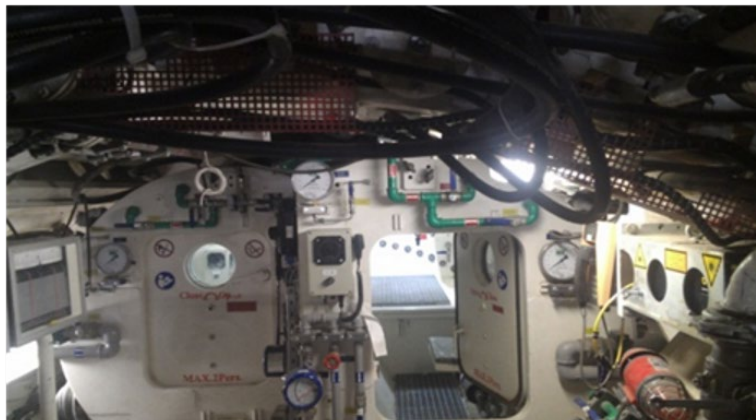
Figure 2 – Airlock shield chamber (Tashkent-2018)
