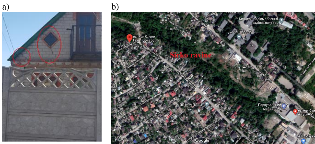
Figure 6 - Deformations of the walls of the house (a) and the position of observation points on the satellite map (b)
