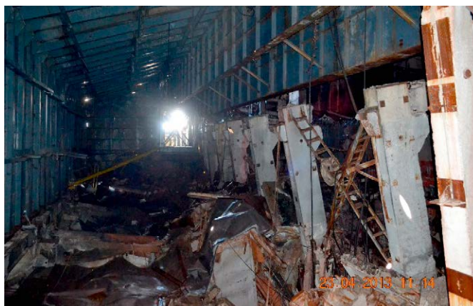
Fig. 11. Current state of the debris at the place of the Mammoth beam temporary support installation
