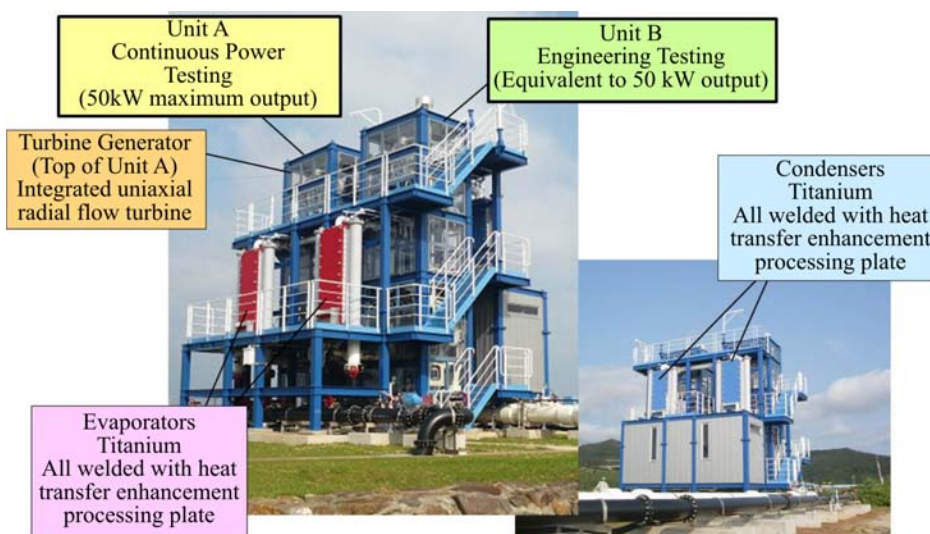
Fig. 2. 50 kW demonstrational OTEC on Kumejima Island [5].
