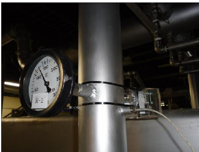
Fig. 10. Installation of TEPG-integrated wireless sensor node device to a pipe.
