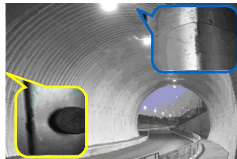
Fig. 1. Damage of zinc coating of metal sheets on the surface of structures of transport facilities.
