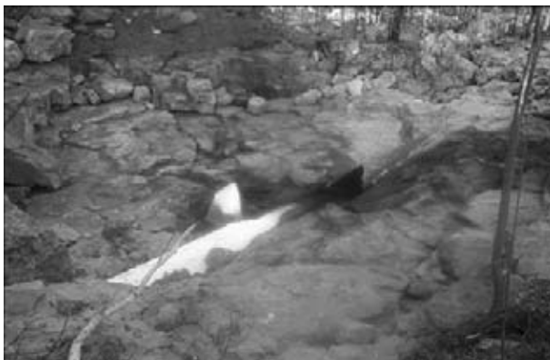
Figure 2. General view of fracture of the main gas pipeline Berge–Yakutsk
