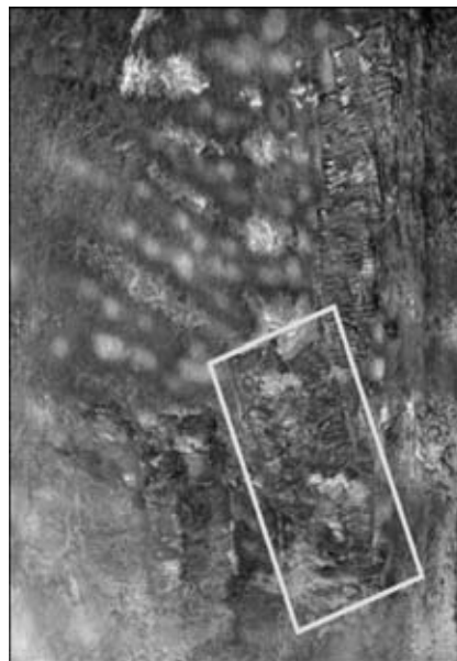
Figure 9. Defects eliminated by cladding on inner steel shell (marked section of the surface, where the network of cracks was rewelded, is shown in Figure 8)
