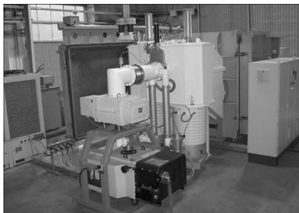
Figure 3. Vacuum system of pumping out of installation ELU-20 with off-line water cooling of vacuum pumps, EB gun and power source («Lahntechnik» chiller of the type BL-365-16, Germany)
