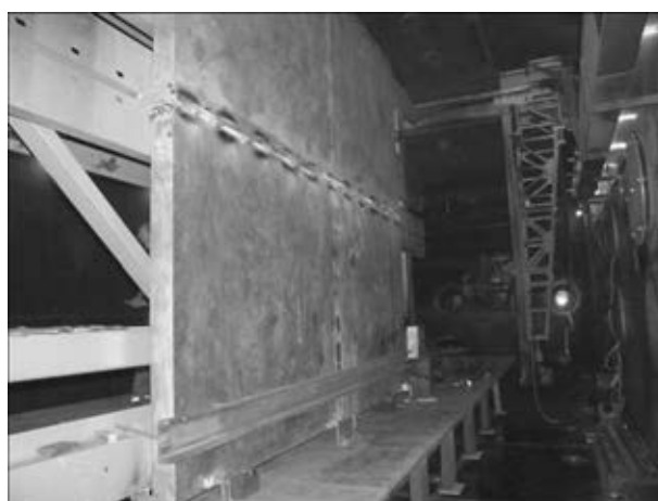
Figure 6. General view of platform of MA2 alloy before making the last weld of 3000 mm length
