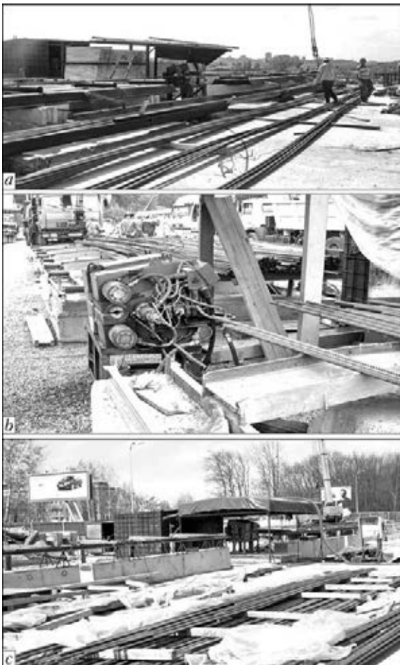
Figure 7. Prototypes of line for reinforcement welding in construction site (a-c — same as in Figure 4)
