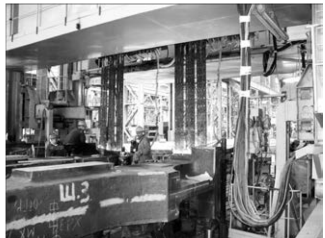
Figure 4. Electroslag welding of two welds by the schematic in Figure 2 (work in progress)
