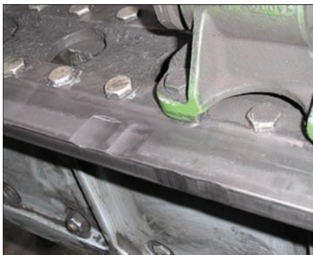
Figure 1. Working surface of rail with worn-out regions
