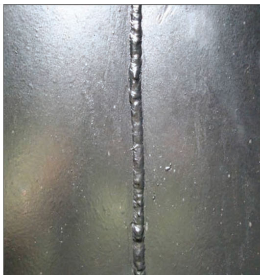
Figure 3. General view of vertical welds on inner wall surface of the main tank
