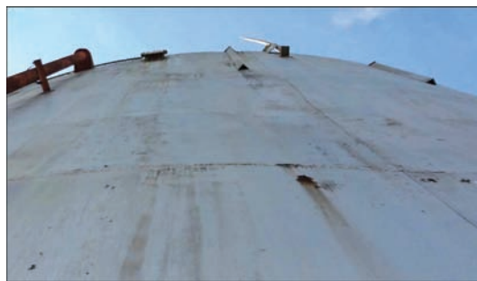
Figure 1. Formation of corrugations and dents on the wall after deployment of coils. 5 thous. m 3 tank with a vertical wall
