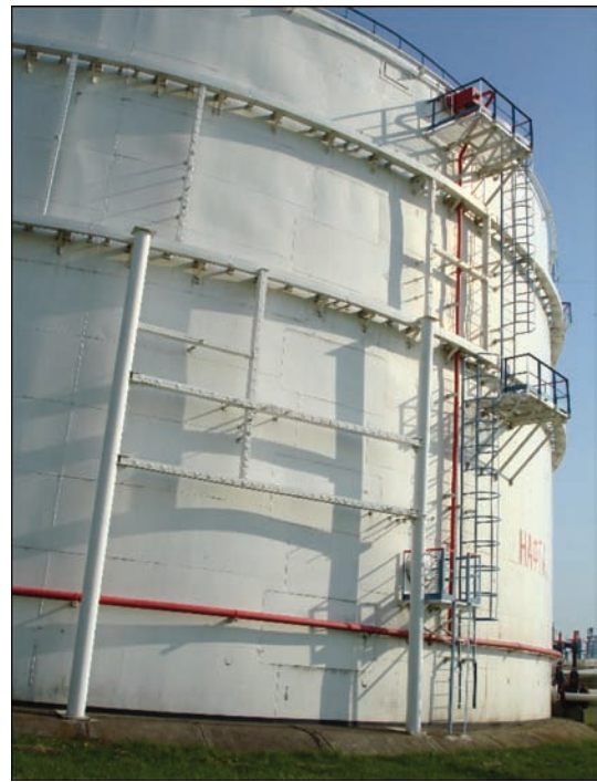
Figure 4. Improvement of geometric shape of the wall of the coiled 20 thous. m 3 capacity vertical wall tank with a fixed roof applying local air holes
