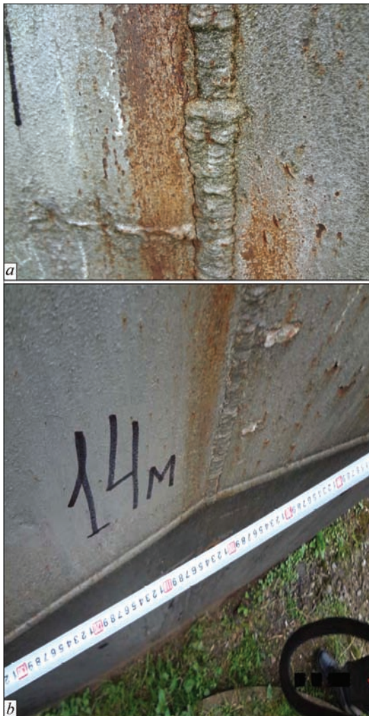
Figure 3. 10 thous. m 3 tank with a vertical wall: fatigue cracks along the weld fusion zone (a); angular deformations in the vertical butt welded joint of the wall (b)
