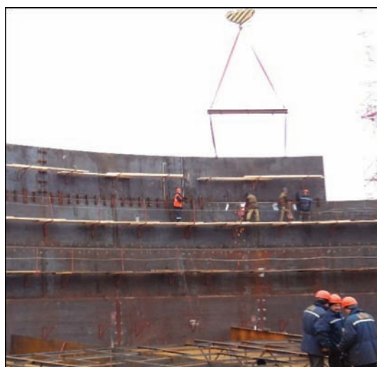
Figure 5. Erection of wall of 50 thous. m^3 vertical wall tank with a floating roof applying sheets of 2.5 \times 8.0 m
