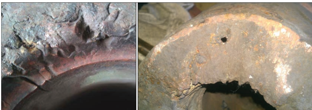
Figure 3. Typical defects of copper chambers after operation
