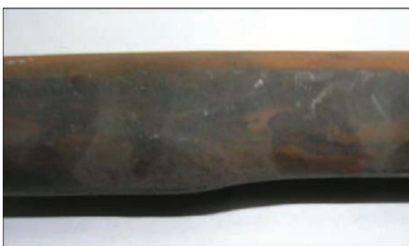
Figure 4. Nature of damage to the FWE tube with a diameter of 32×6 mm as a result of action of ash wear
