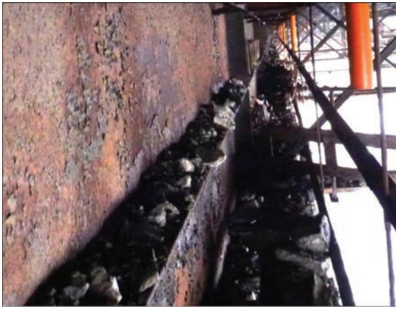
Figure 8. Area of debris accumulation and condition of inspection passages on the inner side of the end beam of the five-span structure
