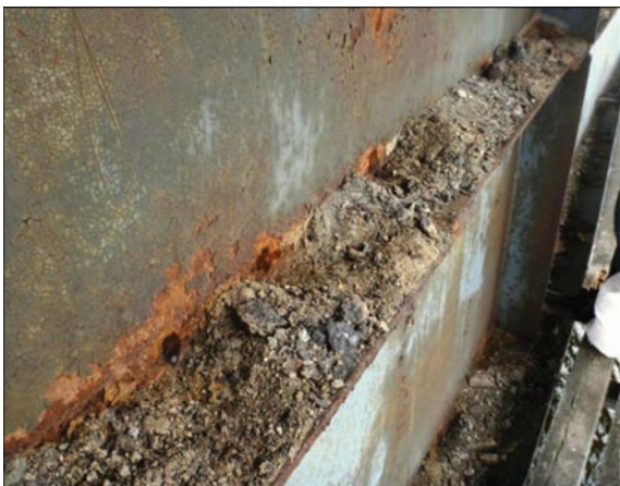
Figure 9. Area of debris accumulation on the outer side of the end beam of the five-span structure
