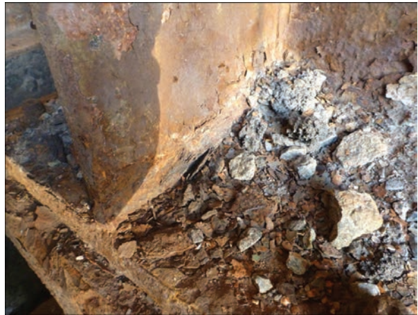
Figure 10. Area of debris accumulation in the supporting part of the four-span structure
