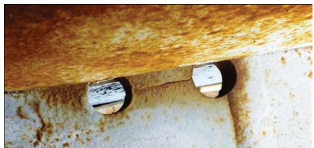
Figure 7. Example of absence of growth of a defect left during erection (ends of the crack were arrested by drilling method) [4]
