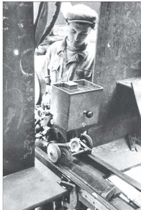
Figure 2. Example of applying automatic submerged arc welding of the lower girth while joining trusses of the main beams [4]
