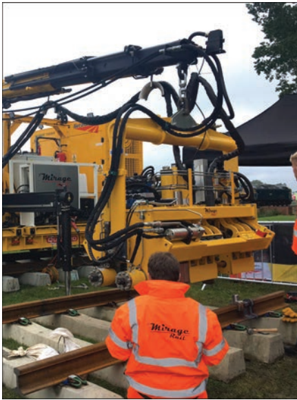
Figure 10. Induction welding robot of Mirage Rail Company of rails is carried out throughout the whole perimeter by the currents of magnetic induction with the help of inductors. The power consumption is 150 kVA.
