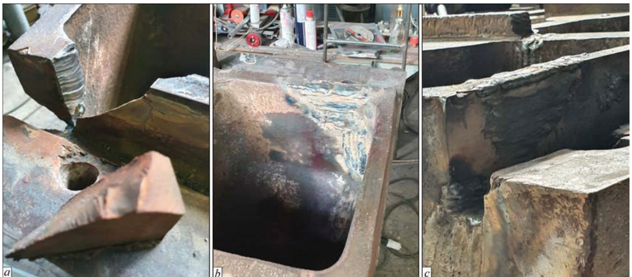
Figure 4. General view of the region of repair of crack No. 1 on the front wall (a), after thermal removal of a wall fragment (b), after welding (c) from the inside and outside, respectively
