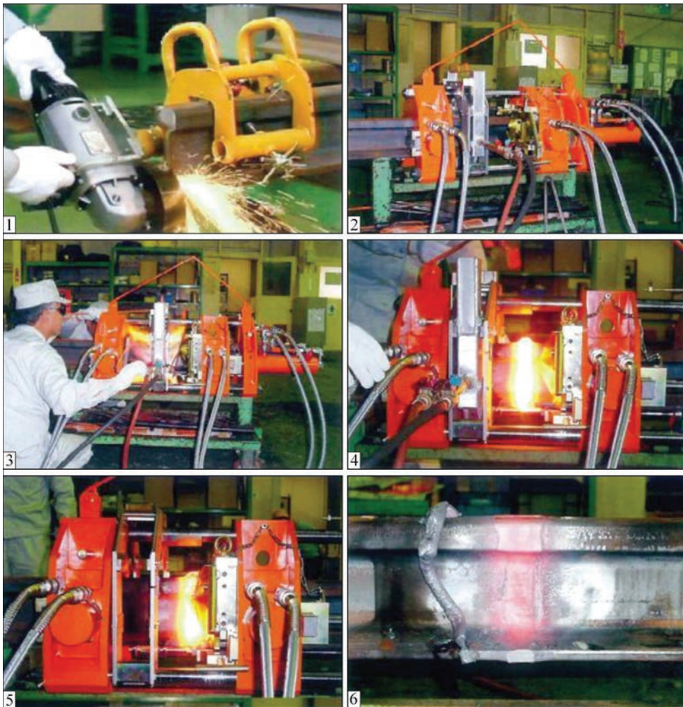
Figure 5. Sequence of technological operations in GPW [19]: 1 — dressing of rail ends; 2 — setting up GPW unit; 3 — GPW process (heating stage); 4 — end of GPW process (upsetting); 5 — flash removal; 6 — welded part immediately after GPW
