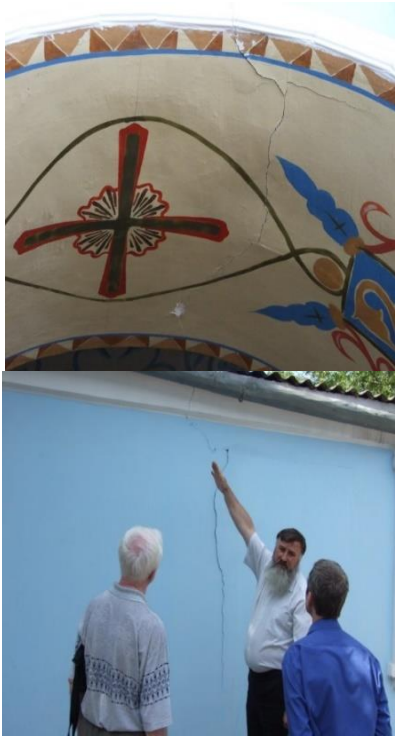
Fig. 2. Church's reaction to the explosion in the quarry. Top – cracks in the brick vault of the Church. Bottom – the priest pointing out vertical cracks on his house located within the Church's premises
