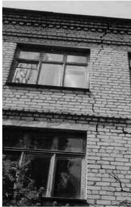
Fig. 3. Visual inspection of School No. 40 revealed cracks up to 0.05 m wide in external load-bearing walls. Crack gauges and vibration monitoring are required to assess seismic and explosion-related impacts
