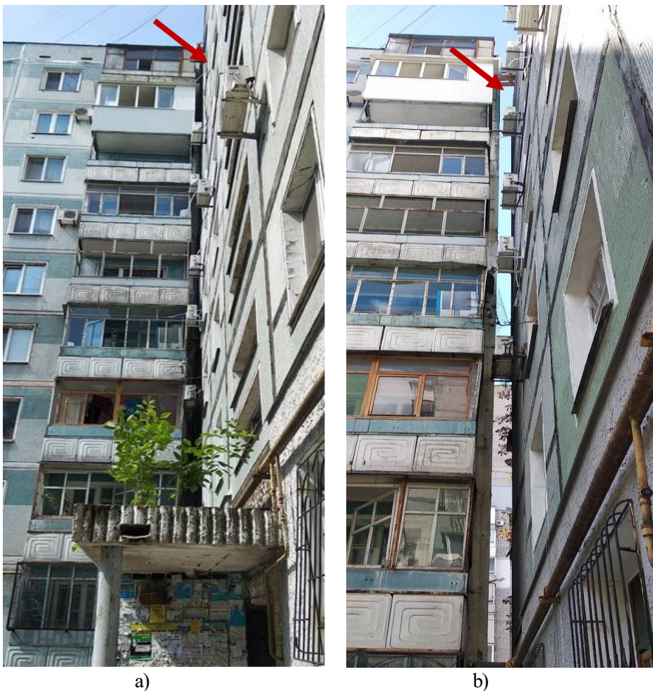
Fig. 9. General view of the deformation seam between block sections No. 3 and No. 1 before straightening (a); and after straightening (b) at 23, 25, Engineer Preobrazhenskyi St., Zaporizhzhya, Ukraine [10]
