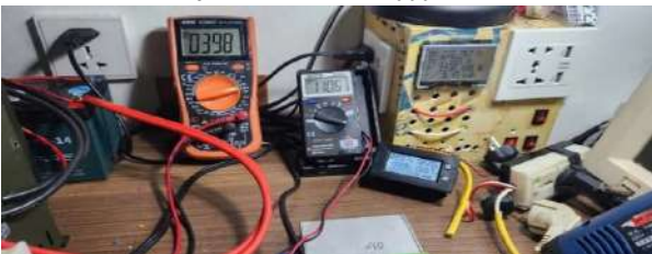
c – AC load near 1500 W
